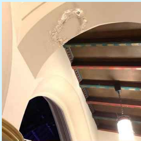
Leaks and Ceilings
