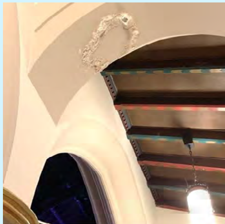
Leaks and Ceilings
